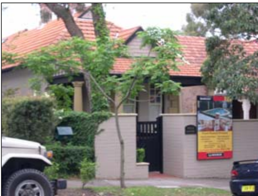
Federation Cottage with inappropriate 'classical' details added such as columns and ashlar quoins.
